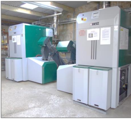
Two sub-200kW Herz FireMatic boilers in the plant room
