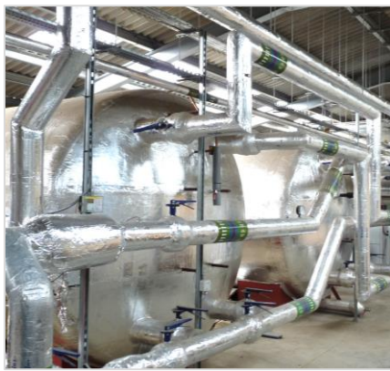
Twin 20,000litre buffer tanks
