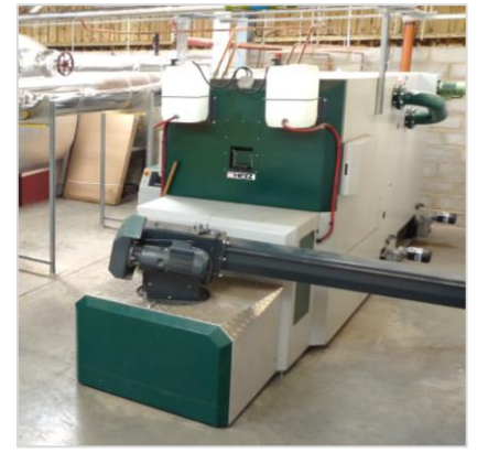
995kW HERZ BioFire boiler
