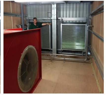
Heat exchangers and fan serving the grain store
