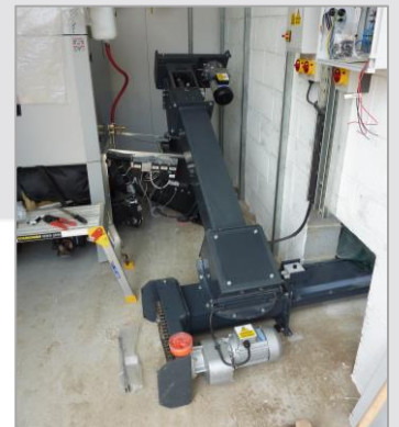
The auger and biomass boiler in the plant room, with an opening to the grain store.
